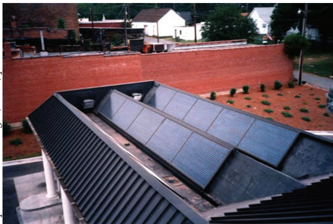
Central Carolina Bank: 2.75 kW e , produces electricity and heats building. Installed in Bessemer City at Central Carolina Bank.
